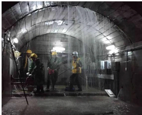
(b) 预制外墙接缝渗漏
