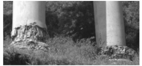
(b) 桥墩底压溃
